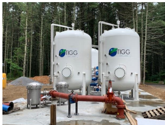
Carbon filter vessels at Cranberry Well
