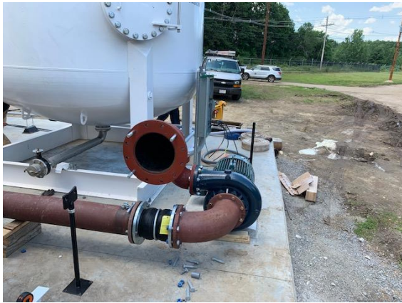
Booster pumps for Chestnut Well
