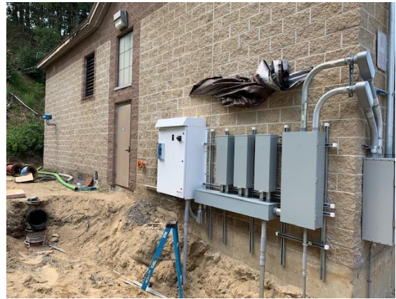
Pump drive & electrical disconnect
