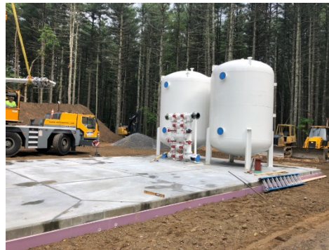
Carbon filter vessels at Cranberry Well
