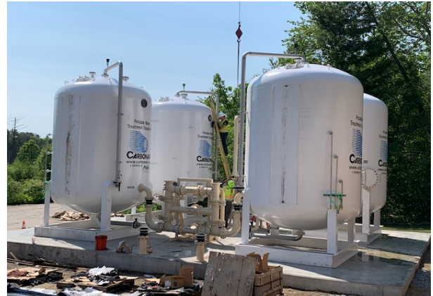
Filter vessels at Chestnut Filtration
