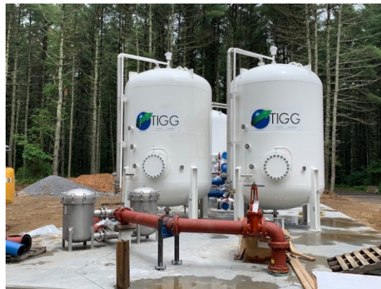
Carbon filter vessels at Cranberry Well
